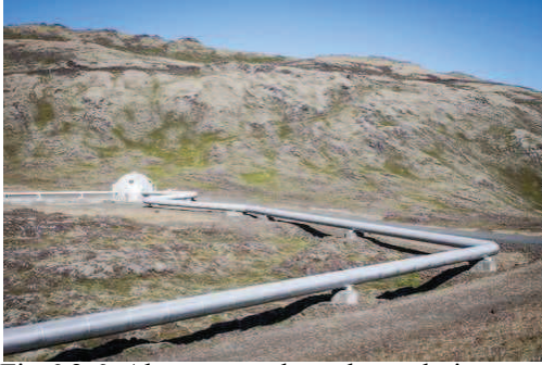
Fig.6.2.6 Aboveground geothermal pipes to the Nesjavellir geothermal power plant
