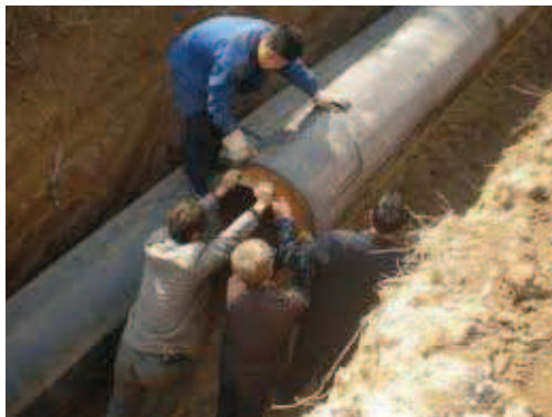
Fig.6.2.7 Buried pre-insulated pipes for geothermal district heating, Xian Yang – China
